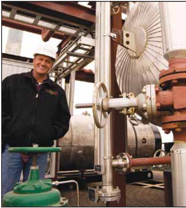
Kevin Baumann, head of Rotex Energy, among the boilers for frac water.
